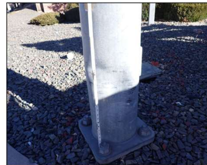
IMPACT DAMAGE ON SOUTHWEST SIDE OF COLUMN
