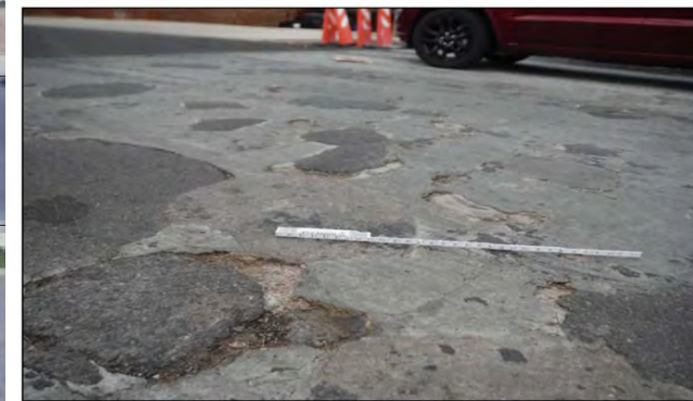
Close up view - Condition of cracking and patchwork in deck surface.
