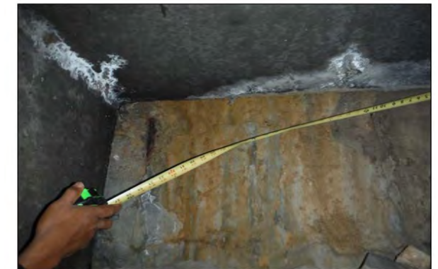
Spalling with exposed corroding rebar in Abutment 2 backwall, Bay C.
