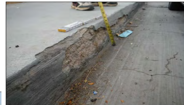
Spalling in East curb face.
