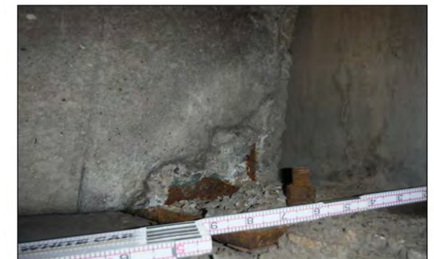
Cracking, spalling with exposed corroding rebar in ends of various girders - Girder 1 at Abutment 2 shown.
