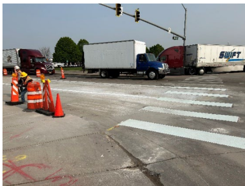
Area of failure
