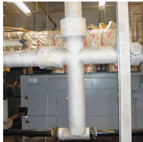
Pipe insulation makes the boiler operate more energy efficiently by allowing the pipes to better retain the hot-water heat.
