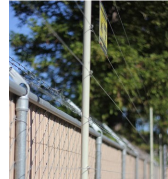
Suspended Wires for Intrusion Detection + Deterrence
