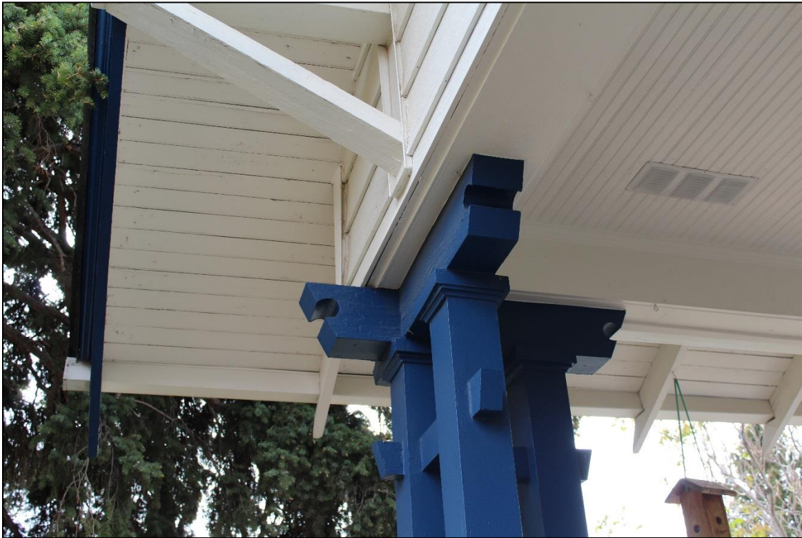
Figure 18: Façade, porch support column. Note the intricate cross-braces. Facing south. Photo: Emma Lane.
