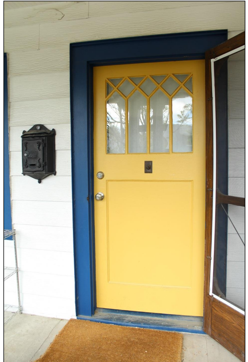
Figure 10: Façade, main entrance. Note the window muntins and historic door ringer. Facing west. Photo: Emma Lane.
