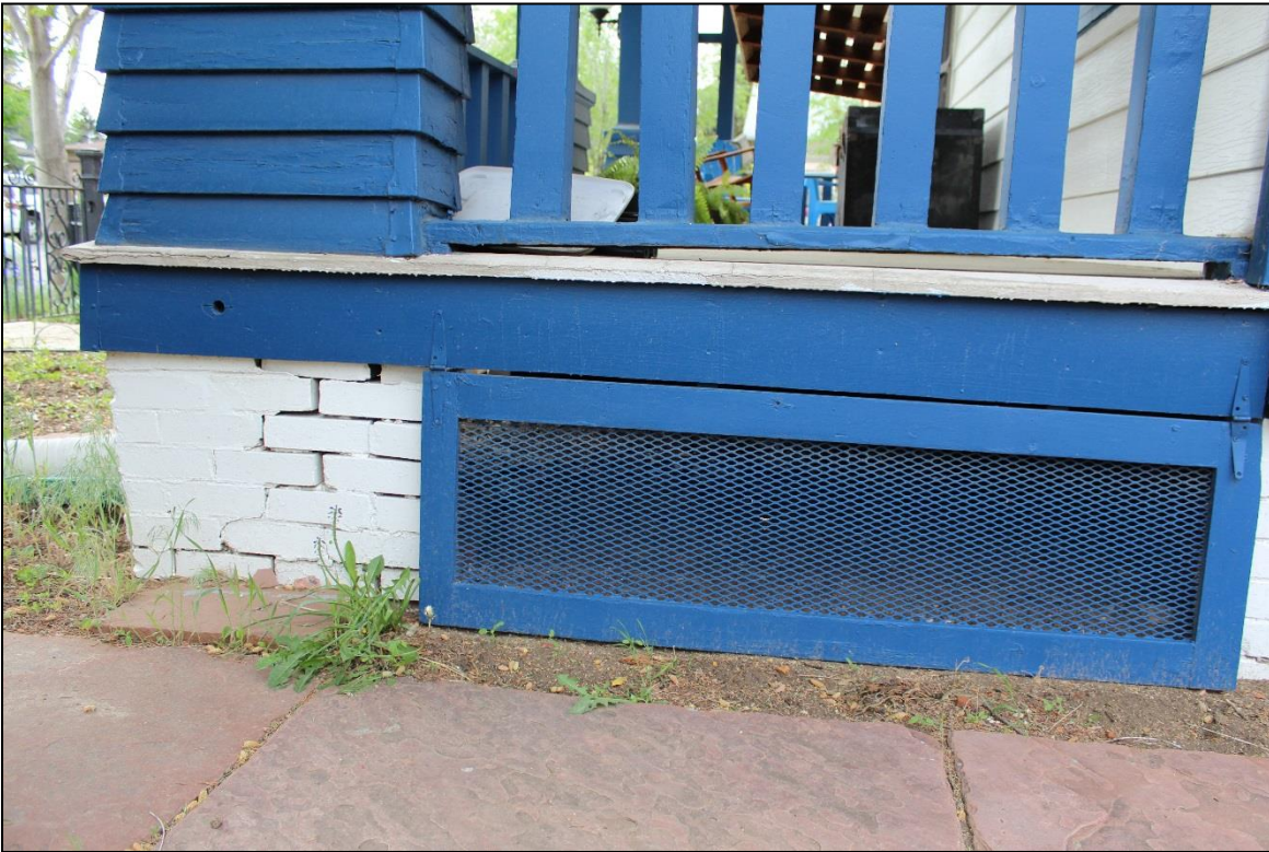
Figure 14: North elevation, porch support foundation. Note the hinged grate. Facing south. Photo: Emma Lane.
