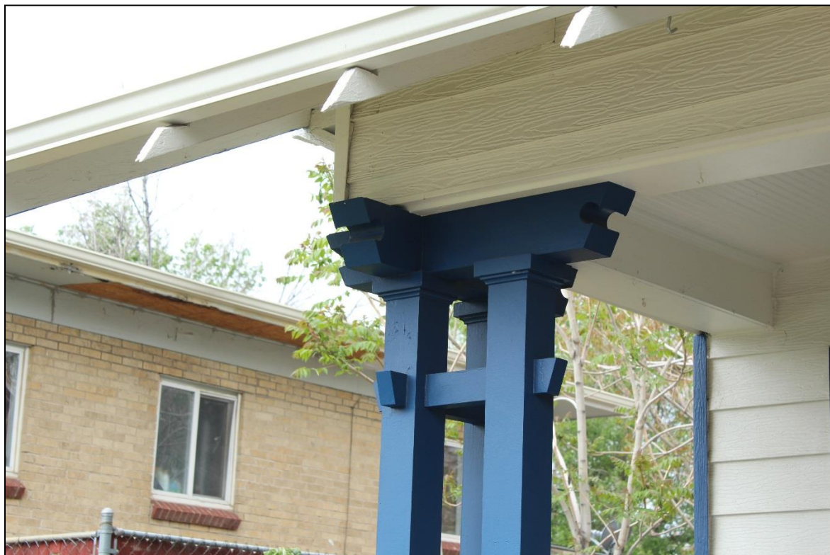
Figure 6: Façade, porch support column. Note the crossbar beams. Facing southwest. Photo: Emma Lane.
