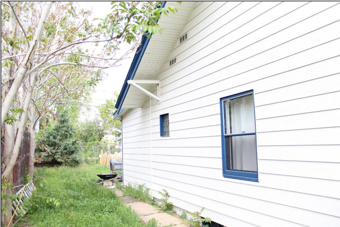
Figure 25: South elevation. Note the overhanging eaves and knee brace brackets. Facing west. Photo: Emma Lane.
