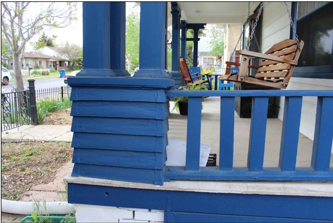
Figure 15: North elevation, porch support foundation. Note the railing. Facing south. Photo: Emma Lane.
