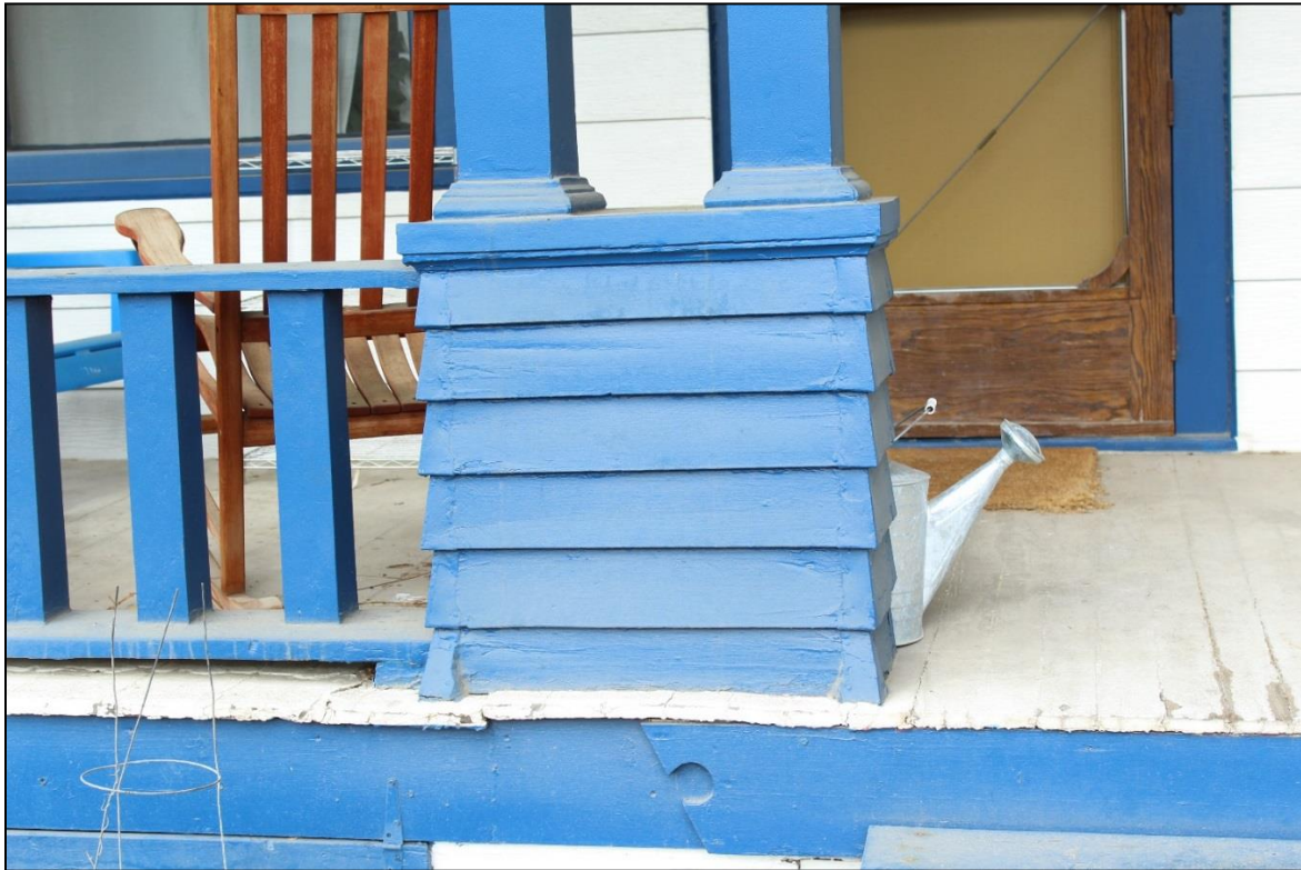
Figure 5: Façade, porch support column. Note the horizontal shiplap siding. Facing West. Photo: Emma Lane.
