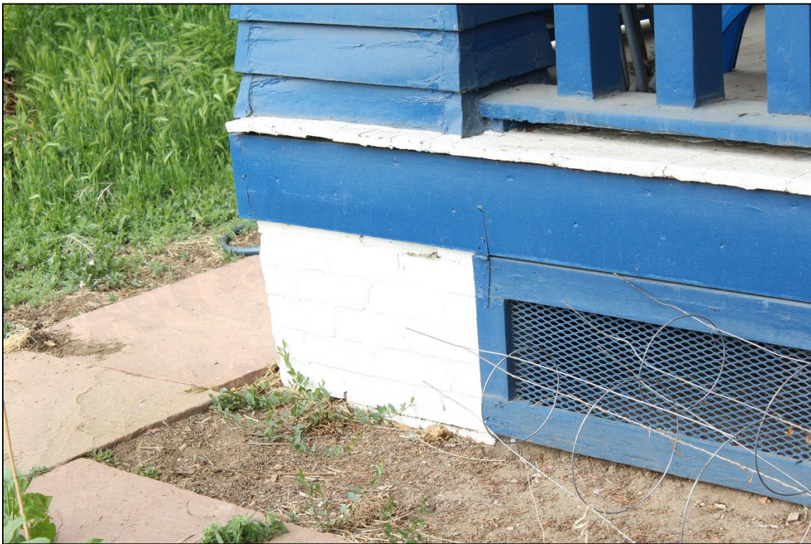
Figure 8: Façade, porch support foundation. Note the hinged grate. Facing southwest. Photo: Emma Lane.
