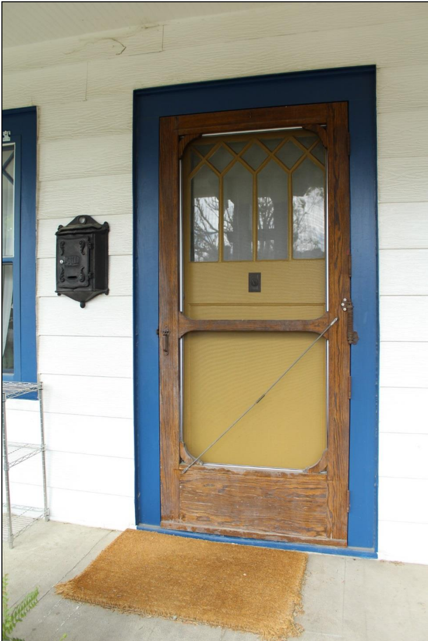
Figure 9: Façade, main entrance. Note the historic screen door and hardware. Facing west. Photo: Emma Lane.
