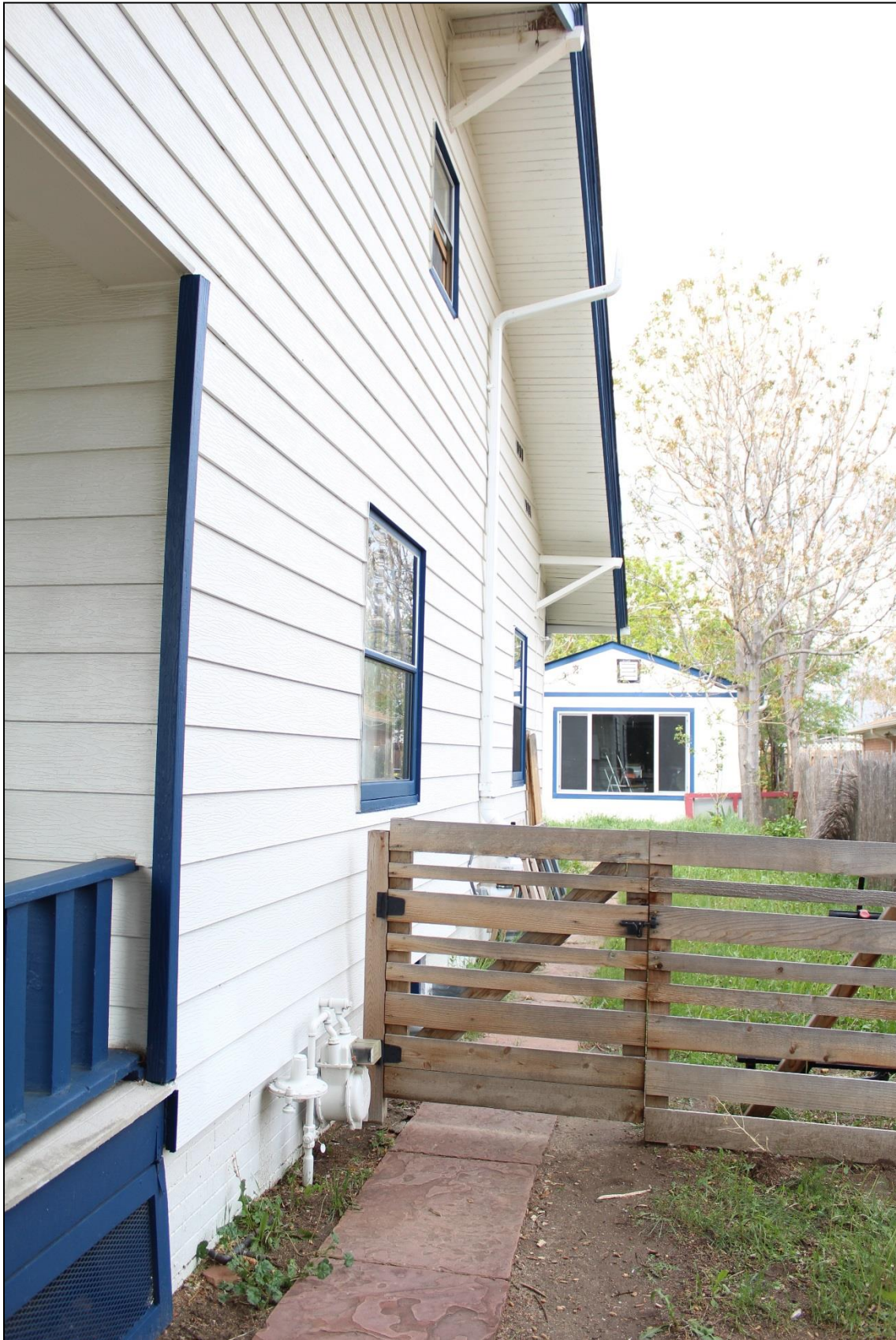
Figure 20: North elevation. Note the overhanging eaves and knee brace brackets. Facing southwest. Photo:
