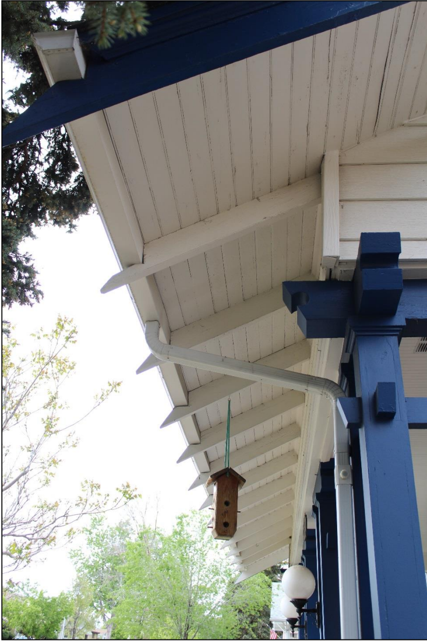
Figure 16: Façade, porch roof. Note the overhanging eaves and stylized rafter tails. Facing south. Photo: Emma Lane.
