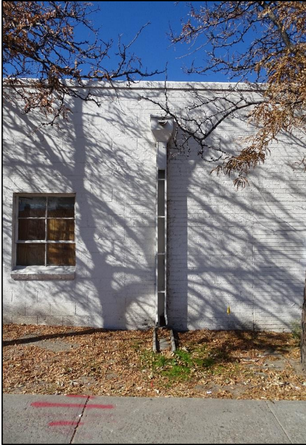
Fig. 11: Strait Lumber Company warehouse gutter, (east elevation), 2018. Photo: Drake Brownfield.
