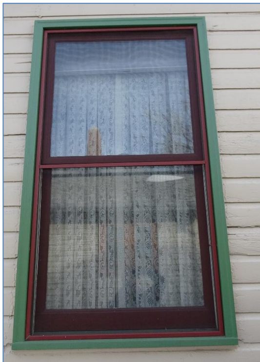
Fig. 18: North elevation, window detail. Note lack of window screen. Photo: Drake Brownfield, 2017
