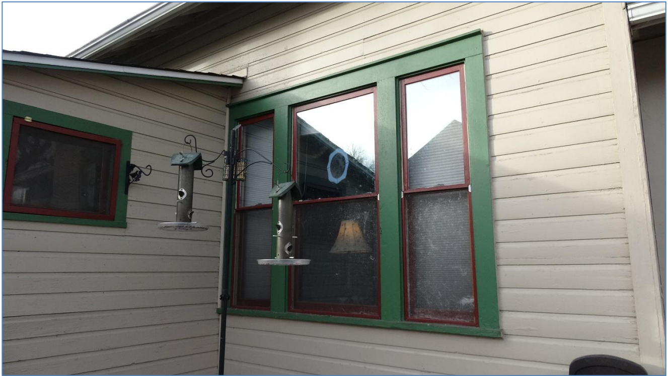
Fig. 20: South elevation, three window ribbon detail. Note various widths and lack of upward window screens. Photo: Drake Brownfield, 2017
