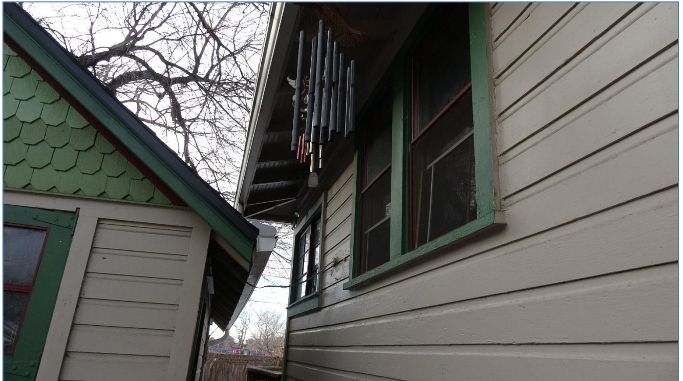
Fig. 25: South elevation (at SW corner), kitchen bump-out detail. Note window ribbons. Photo: Drake Brownfield, 2017
