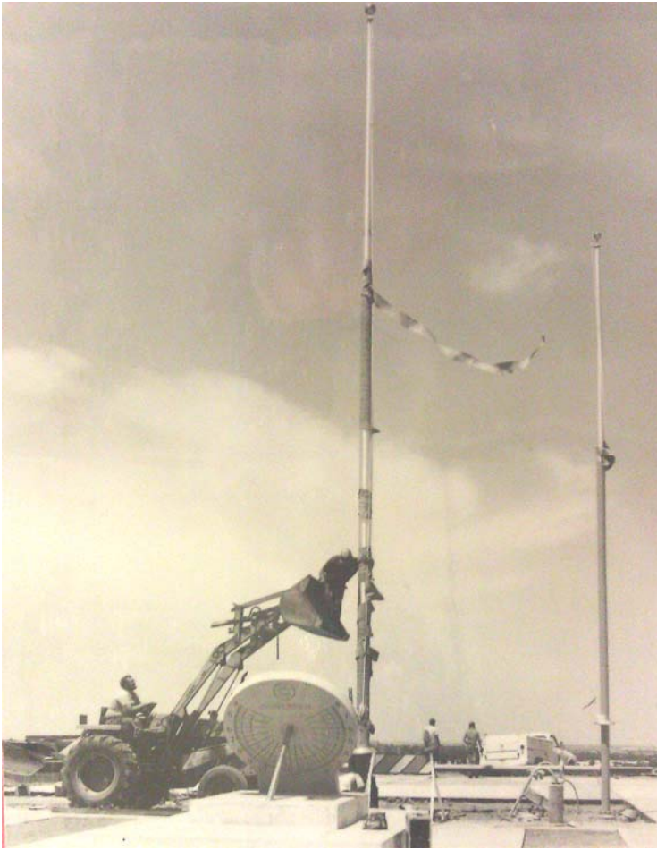
Figure 13. Erecting flag pole at Bicentennial Park. Note original Lowry Building 1600. View looking north. Photograph courtesy Aurora History Museum archives.
