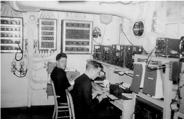
Figure 6. Interior of a Navy radio control room.
