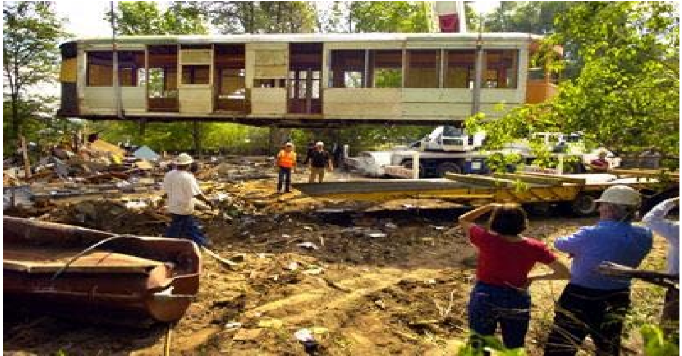
Weitz Construction supervises the lifting of the Trolley Trailer No. 610 from the remains of the Perrott farm house, July 2006.
